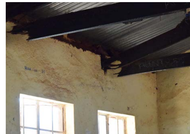
■ Many of the schools in Malawi are poorly constructed and are dangerous. This image shows several broken roof trusses. Quite a contrast to how Kuwala's Campus is built! Kuwala_2024
