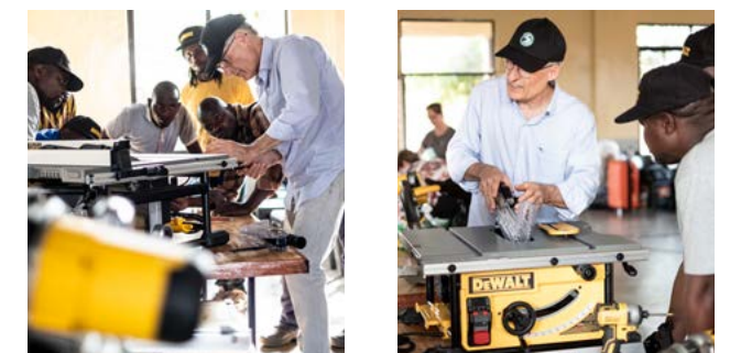
■ DeWalt table saw installation in the workshop. Kuwala_2024
