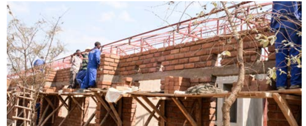
■ The walls and the roof trusses going up on the third hostel.. Kuwala_2024.
